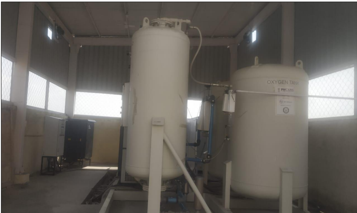
PSA Oxygen Plant of 1000 LPM capacity for augmentation of Oxygen supply efforts
